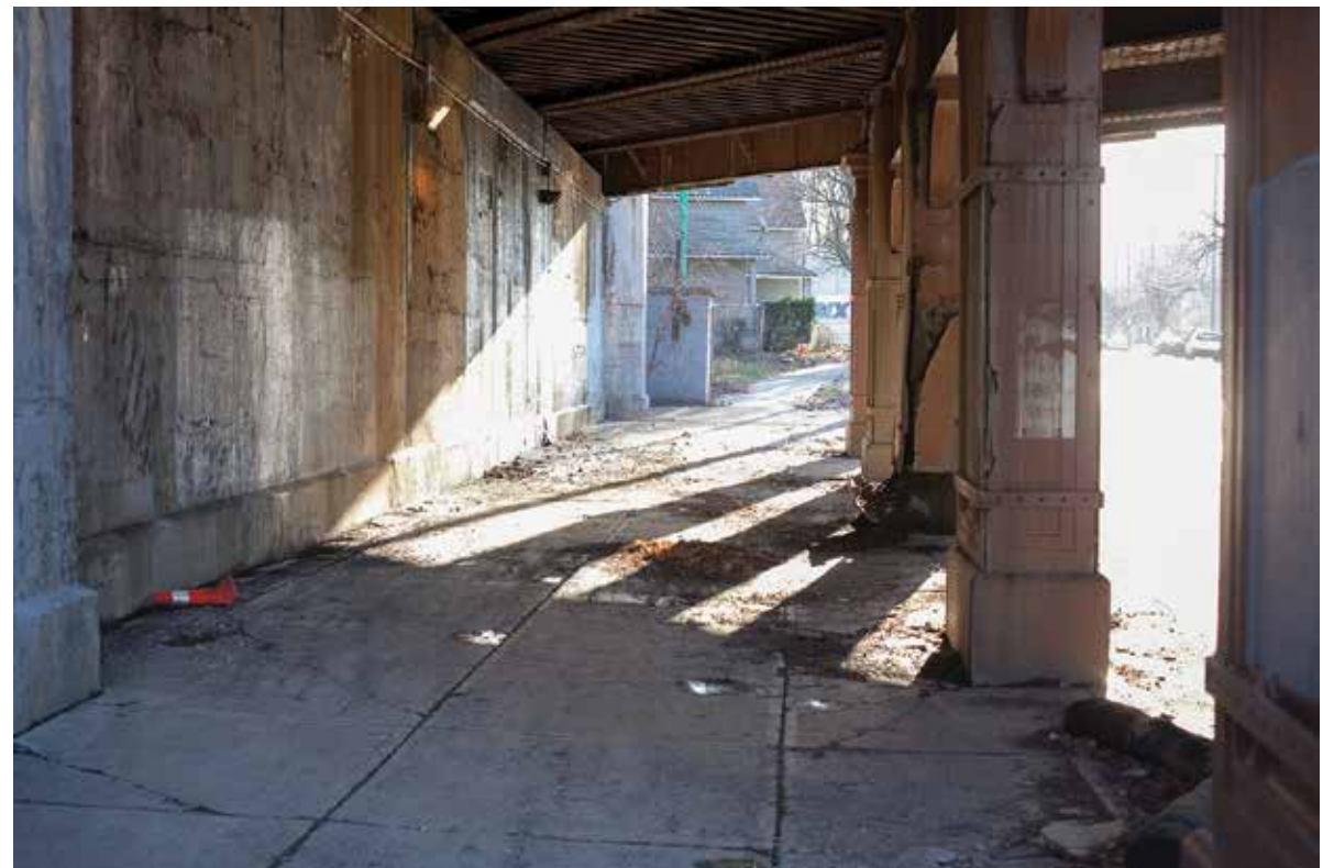
PHOTO BY JULIA VAN WAGENEN February 27, 2018; Lake Avenue between W. 87 th and Clifton: The underside of the Lake Avenue Bridge with pieces of concrete and metal from the bridge that have fallen on the sidewalk beneath the bridge.
